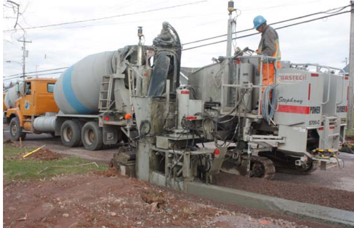
Workers install curbing on Willow Street earlier this fall. The Willow Street infrastructure renewal project has been put on hold until next spring. (Tom McCoag/Town of Amherst)
