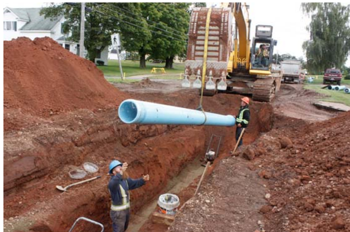
Workers from Beale and Inch Construction Ltd. replace the water main on Willow Street earlier this fall. Work on the Willow Street infrastructure project has been placed on hiatus until next spring. (Tom McCoag/Town of Amherst)
