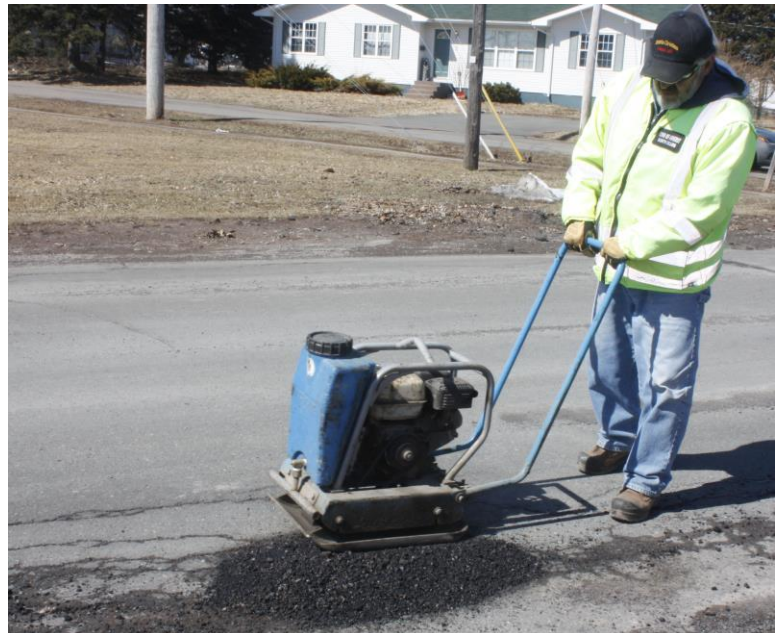
Dusty Collins operates a vibrating compactor while repairing a pothole on Park Street. (Tom McCoag / Town of Amherst)
