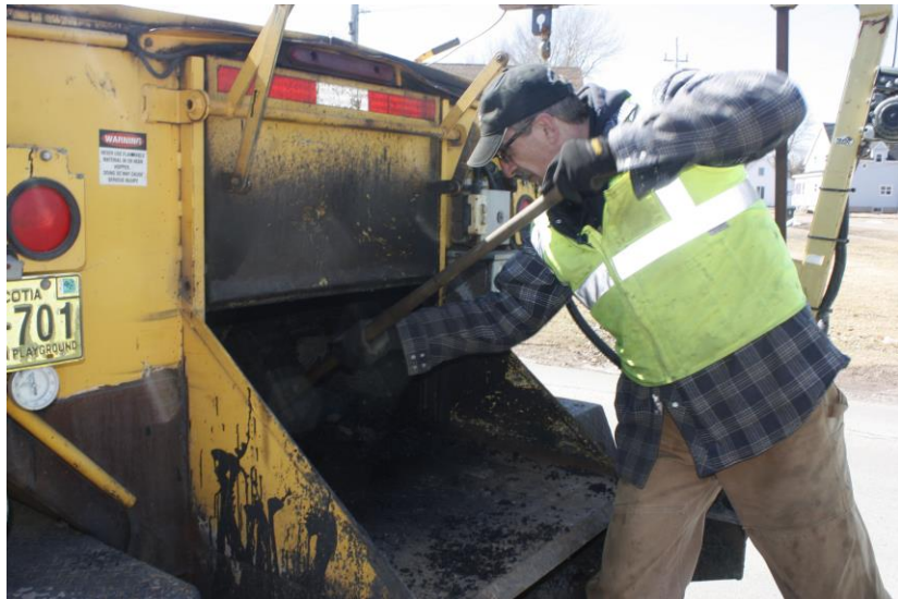
Lester Fromm drives his shovel into a hopper full of heated recycled asphalt as he works to repair potholes. (Tom McCoag / Town of Amherst)
