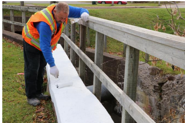
Town employee Vaughn Martin, a master mason, is doing the masonry work at Christie Park. (Tom McCoag / Town of Amherst)
