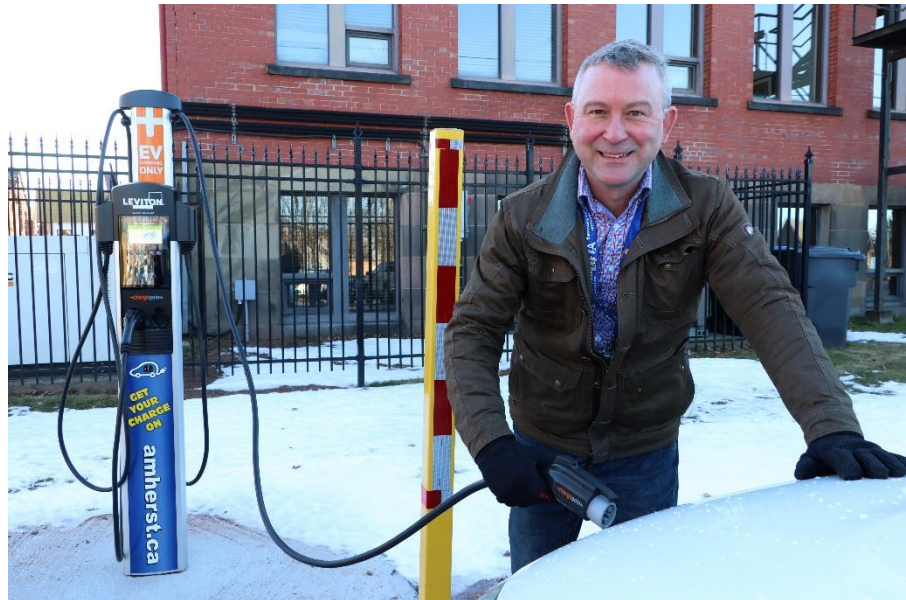
JEFF BACON, BUSINESS DEVELOPMENT OFFICER FOR THE TOWN OF AMHERST, USES THE NEW LEVITON CHARGING STATION TO CHARGE AN ELECTRIC-POWERED VEHICLE. THE CHARGING STATION HAS BEEN INSTALLED BEHIND THE AMHERST TOWN HALL. (TOM MCCOAG / TOWN OF AMHERST)
