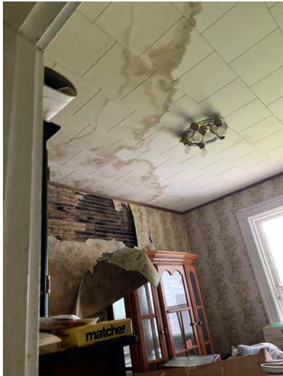
Main floor water damage.
