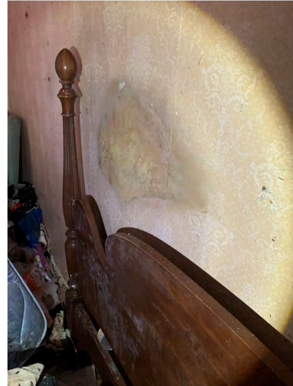
Second-floor bedroom. Light appeared to scorched wallpaper.
