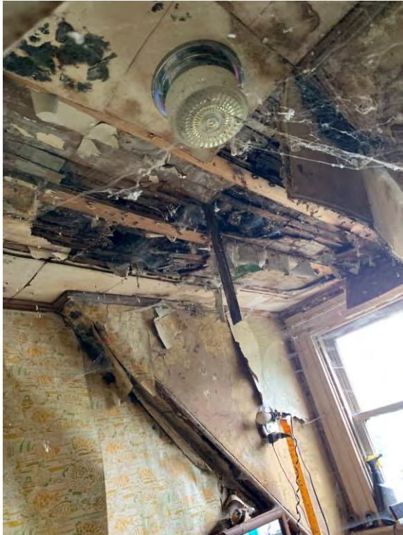
Second-floor bathroom water damage.
