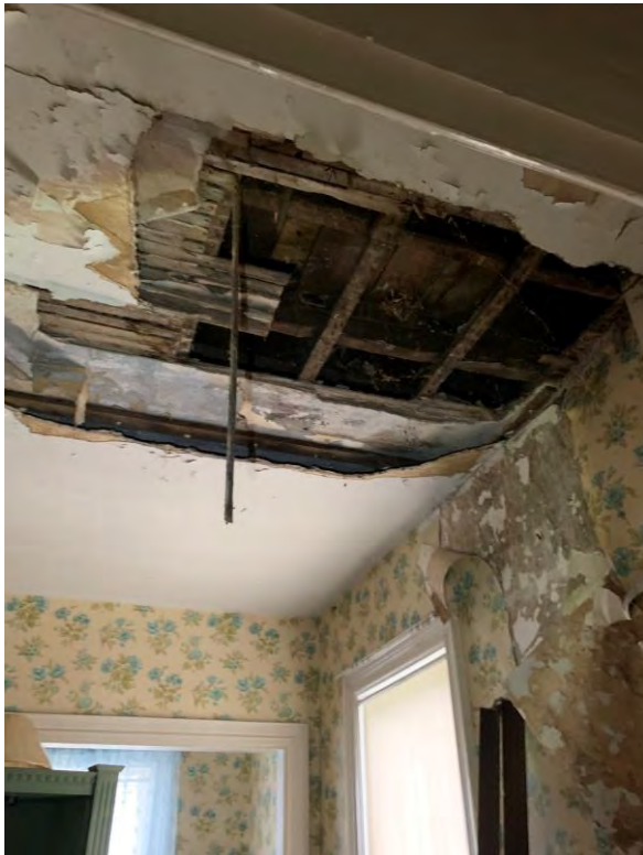
Second-floor water damage.
