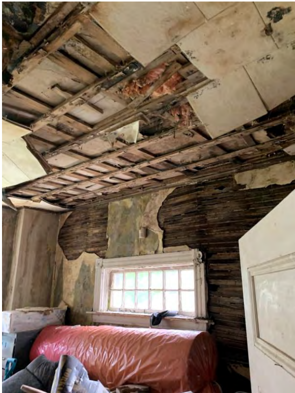
Main floor water damage.
