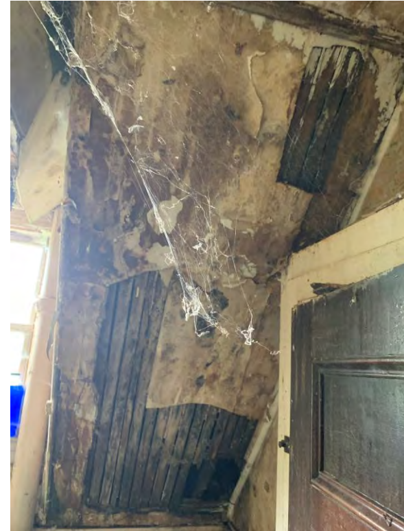
Second-floor water damage.
