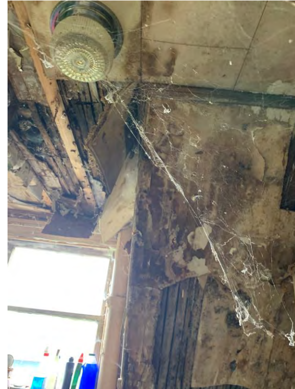
Second-floor bathroom water damage.
