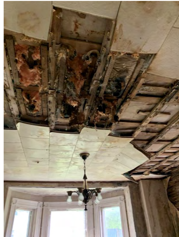
Main floor water damage.
