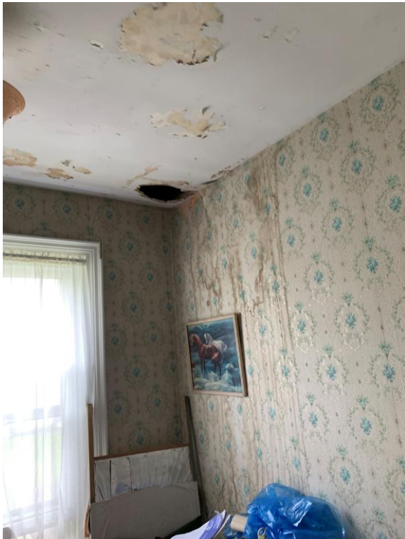
Water damage on second-floor.
