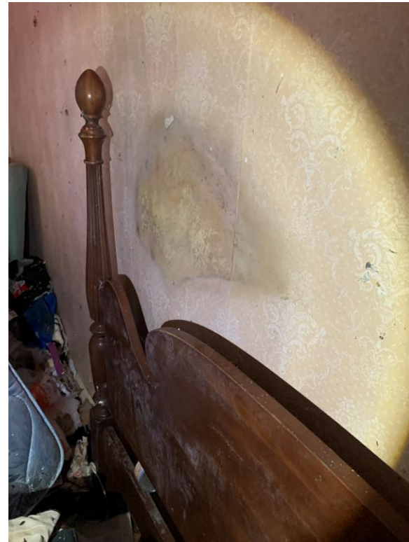
Second-floor bedroom. Light appeared to scorched wallpaper.
