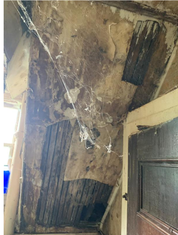
Second-floor water damage.
