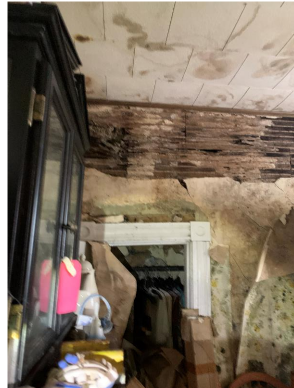
Main floor water damage.
