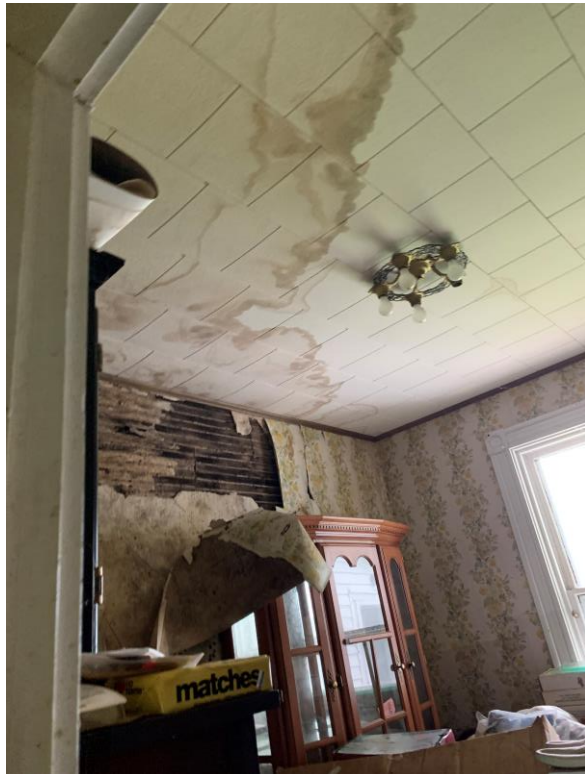
Main floor water damage.
