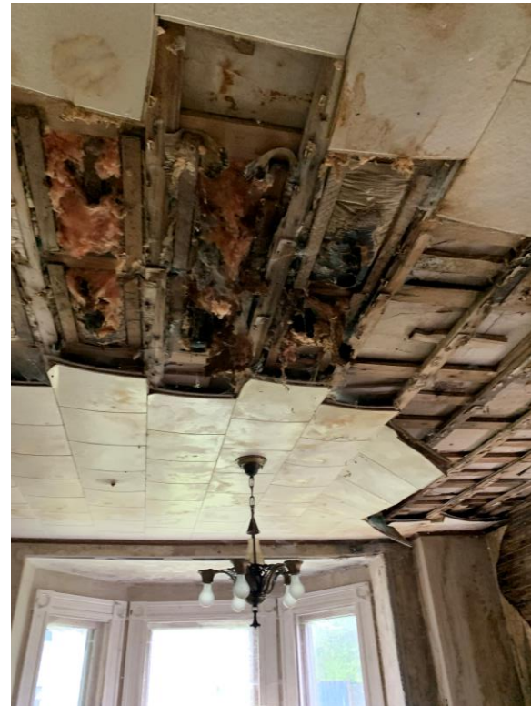
Main floor water damage.
