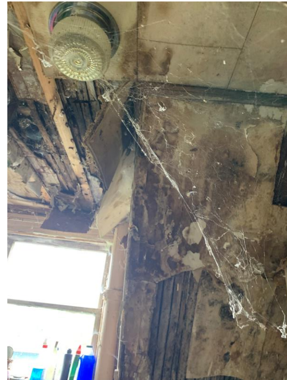
Second-floor bathroom water damage.
