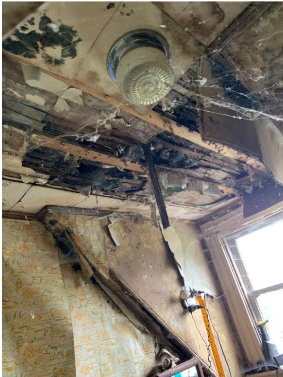
Second-floor bathroom water damage.
