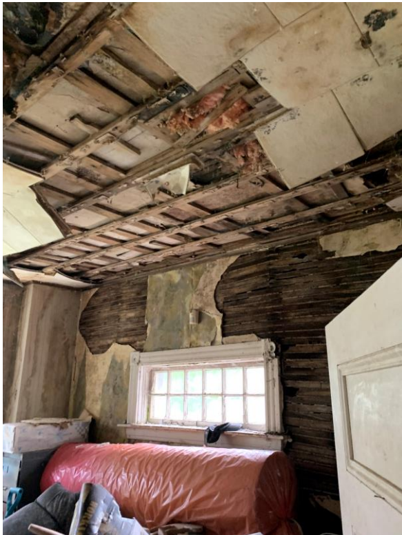
Main floor water damage.
