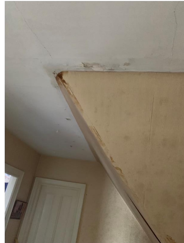
Minor water damage on second-floor.
