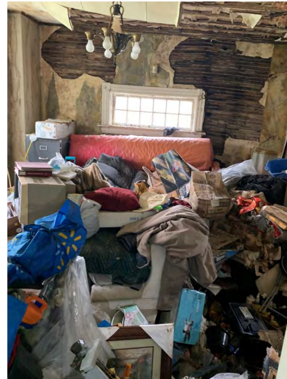
Main floor water damage, hoarding.
