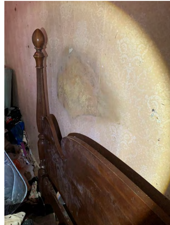
Second-floor bedroom. Light appeared to scorched wallpaper.
