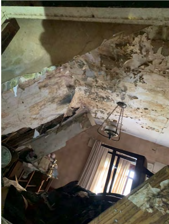
Second-floor water damage.
