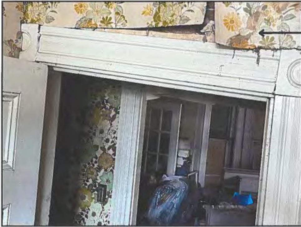
Slanted door frame due to active settlement. Approximately 3 1/2" of settlement in a 3'-0" run
