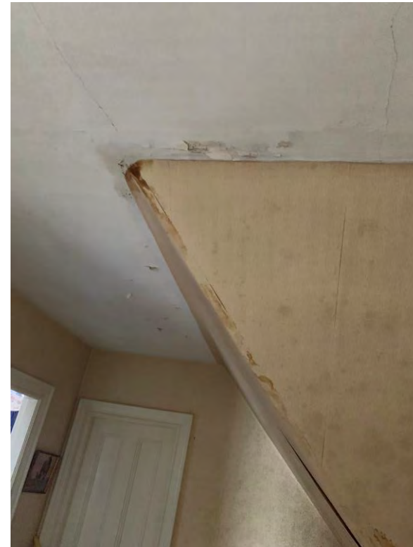
Minor water damage on second-floor.
