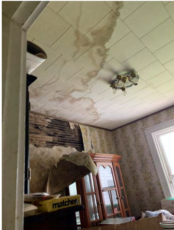
Main floor water damage.
