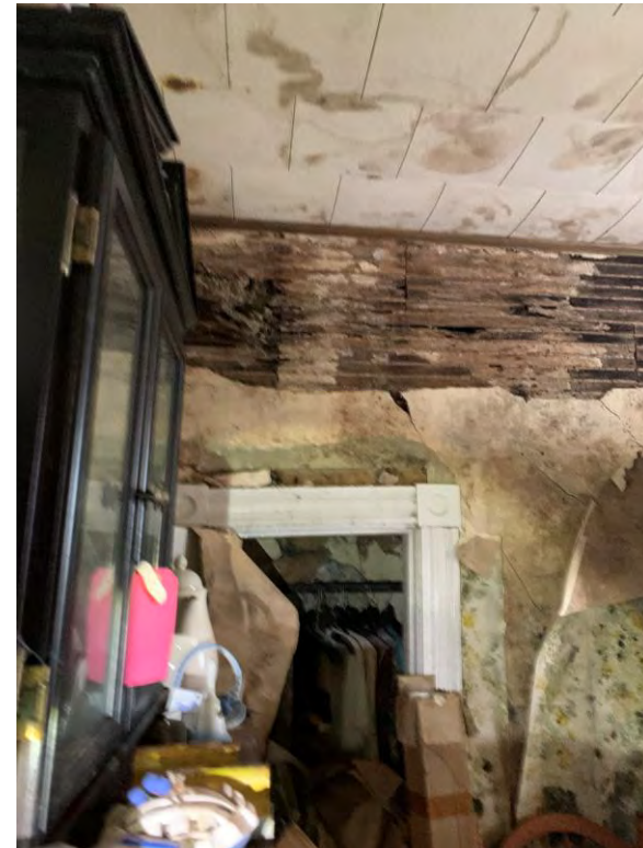
Main floor water damage.
