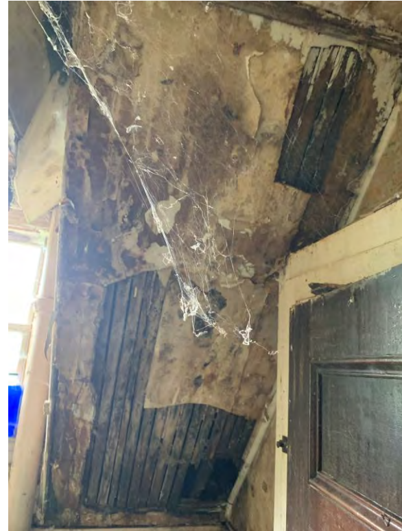
Second-floor water damage.
