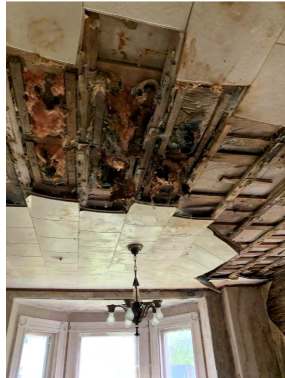
Main floor water damage.
