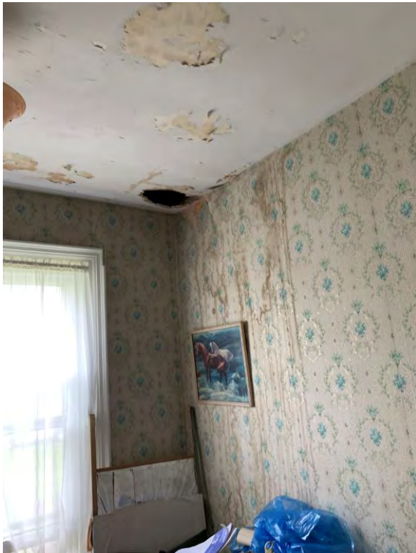
Water damage on second-floor.
