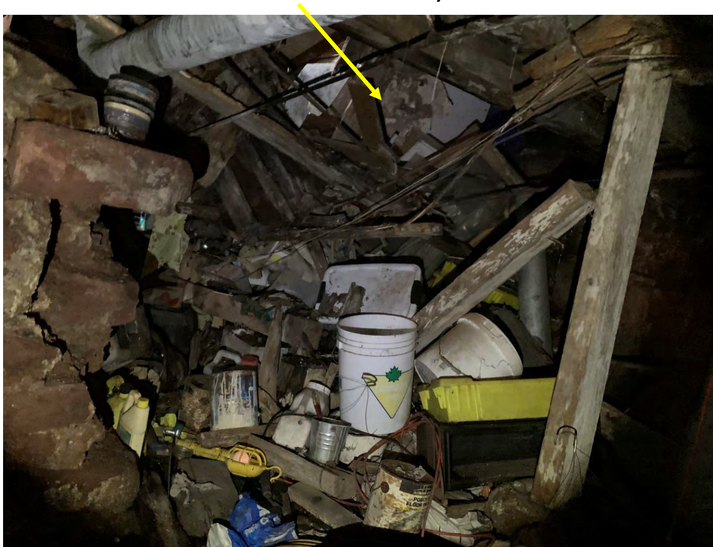
Kitchen has collapsed into basement and little to no floor remains (refrigerator has fallen into the basement)
