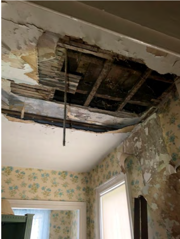
Second-floor water damage.
