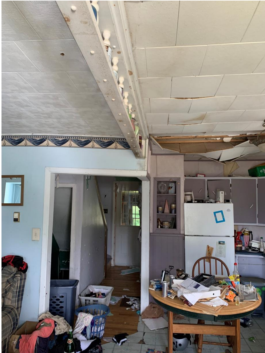
Wall/ceiling starting to sag
