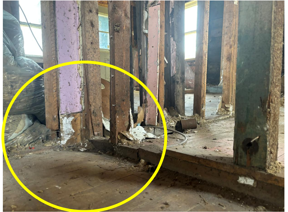
Significant sag – possible broken support beam
