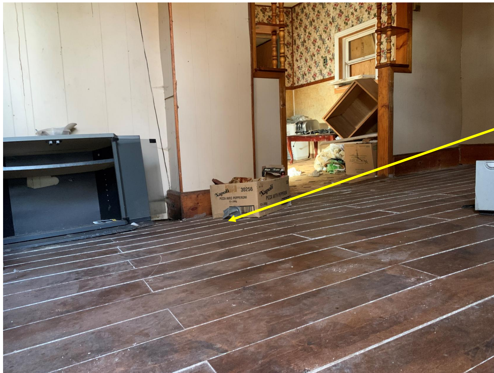
Significant bowing in floor
