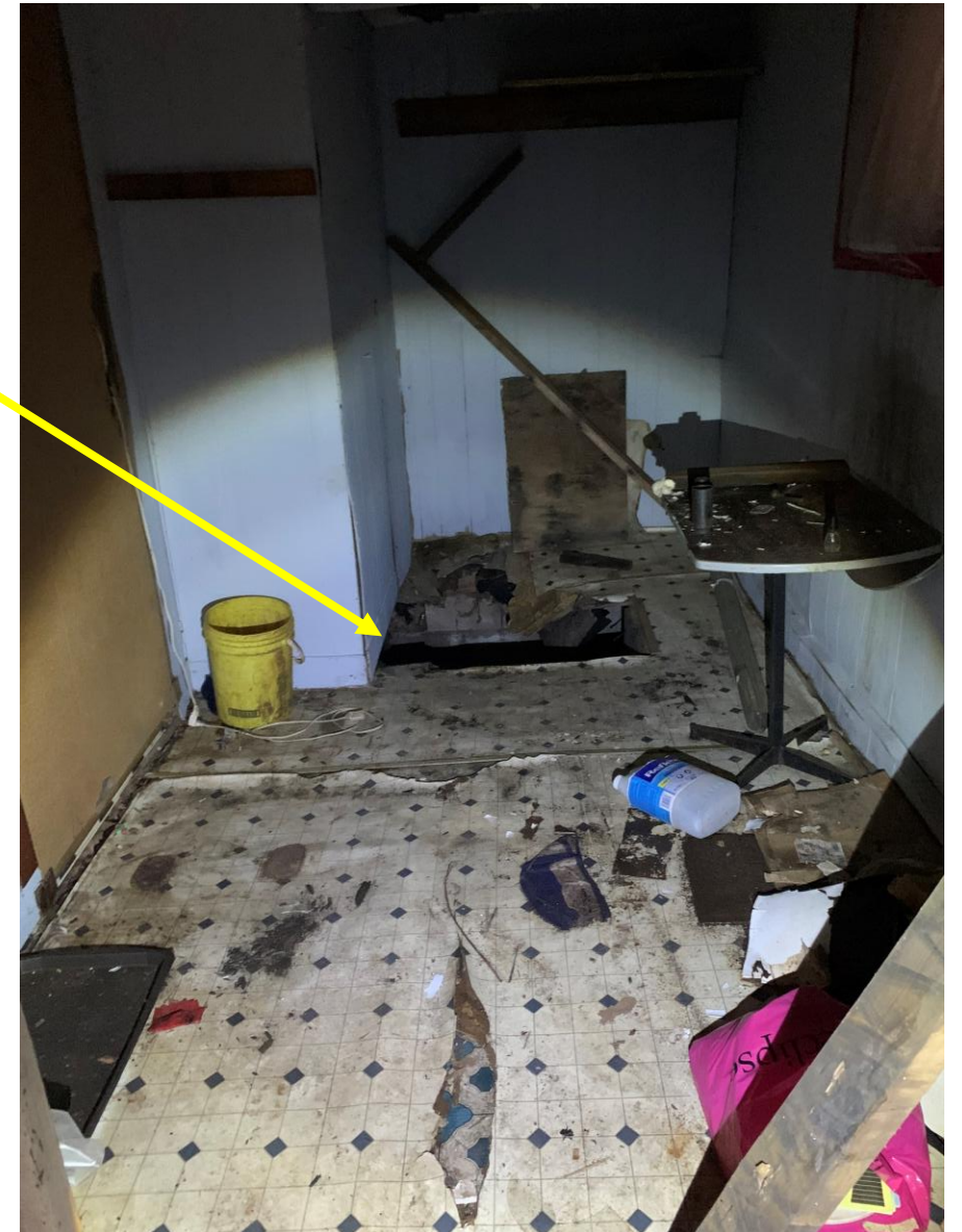
Hole in floor of back portion of building
