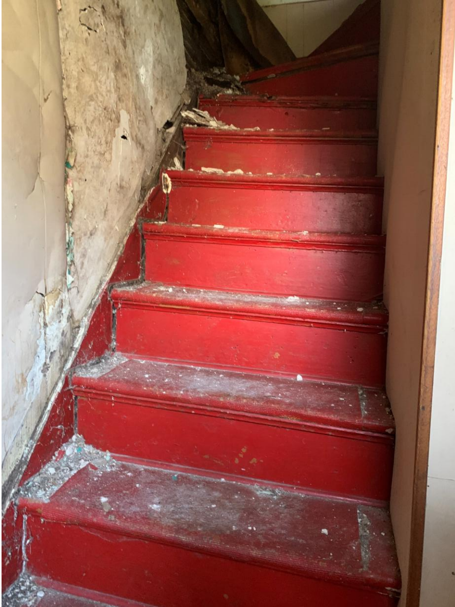
Stairs to second floor are leaning inwards
