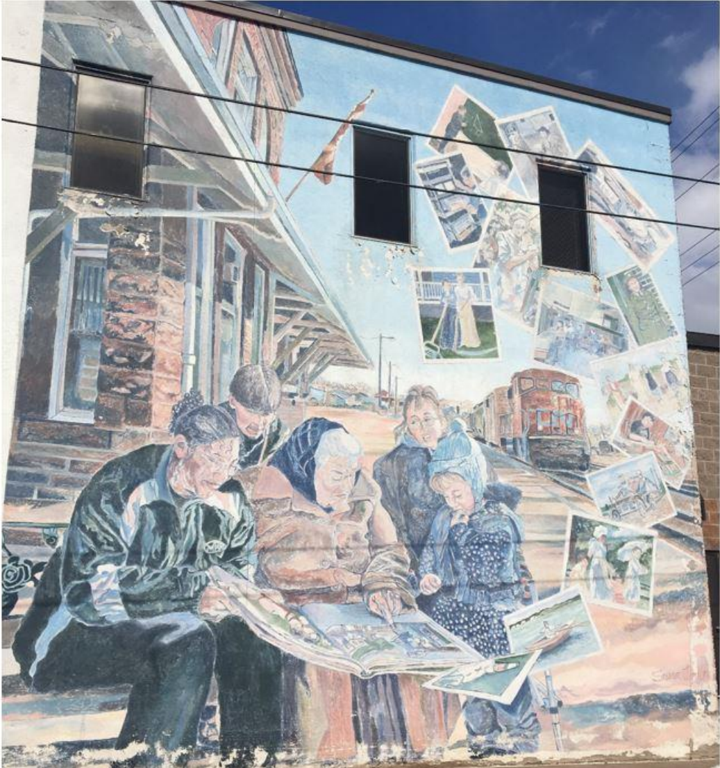
Located at 26 Prince Arthur St. this mural was painted directly on the side of the building by Susan Tooke in 2002. It is beginning to peel in several areas, most noticeably along the bottom of the building and directly under windows. It is in fair condition.
