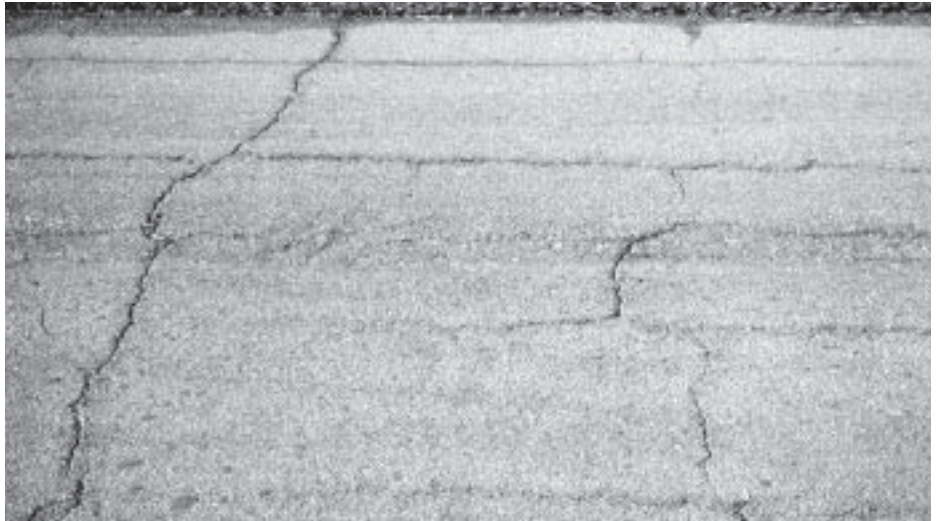
▼ Block cracking with open cracks.
