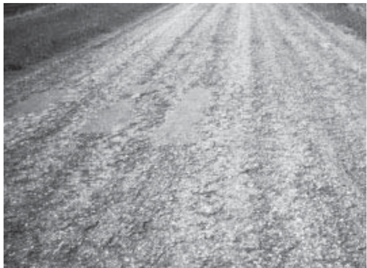
◀ Severe raveling and loss of surface material.
