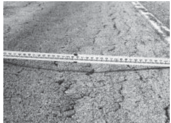
▲ Severe rutting. Strengthen base and reconstruct.
