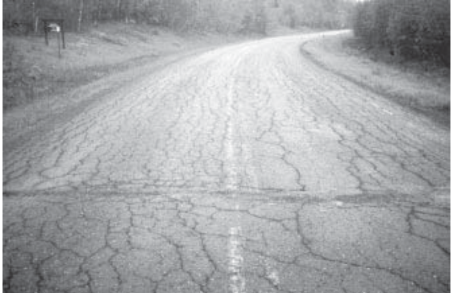
► Extensive alligator cracking. Pulverize and rebuild.
