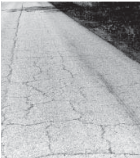
▲ Extensive block cracking in an irregular pattern.
