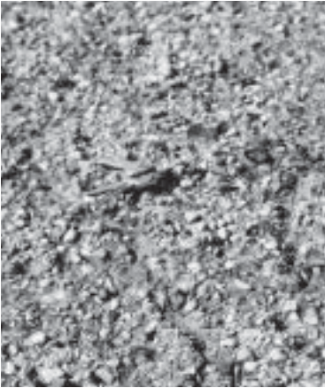
Severe raveling with ▼ extreme loss of aggregate.
