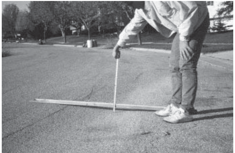
► Severe settling from utility trench.
