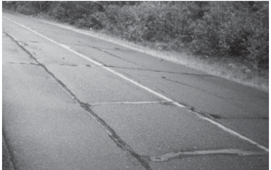
► Concrete joints reflected through bituminous overlay.
