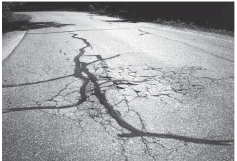
► Frost heave damage from spring break-up.
