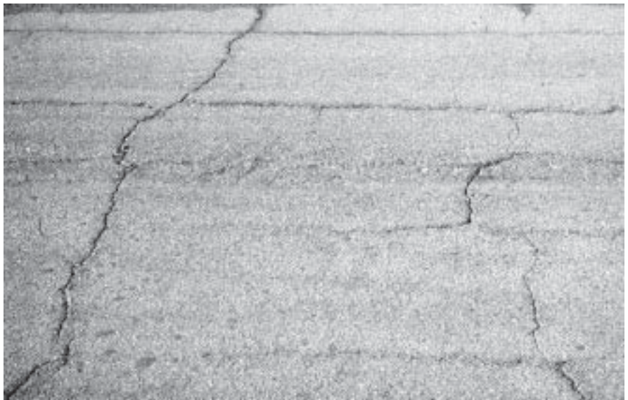
▶ Intermediate-size block cracking, 1'-5' across with open cracks.
