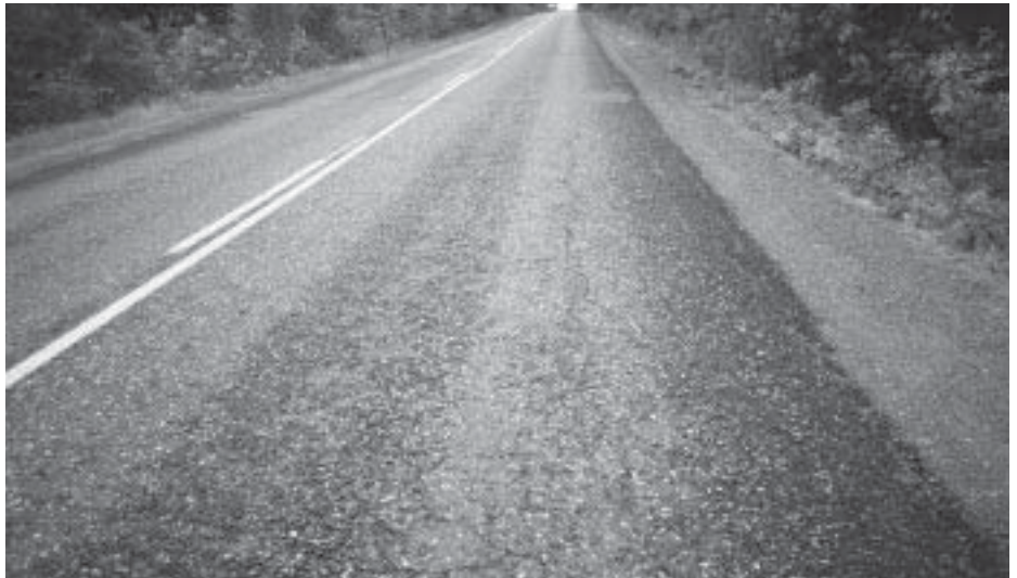
► Moderate to severe raveling in wheel paths.
