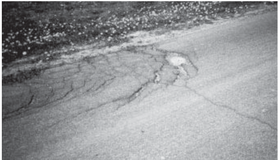
► Crescent-shaped cracks characteristic of slippage.
