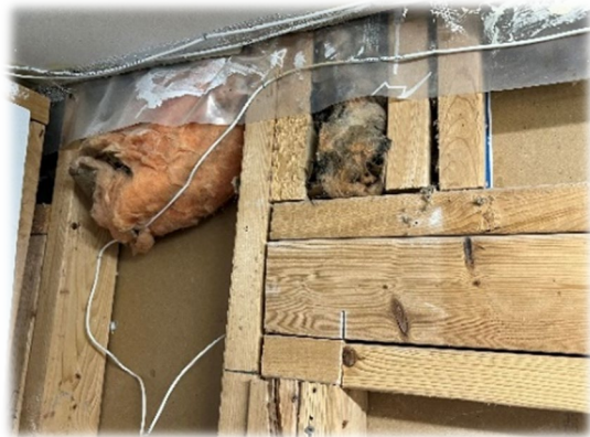
Poorly insulated Interior walls
