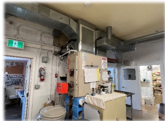
Furnace room and central area for laundry and animal washing stations
